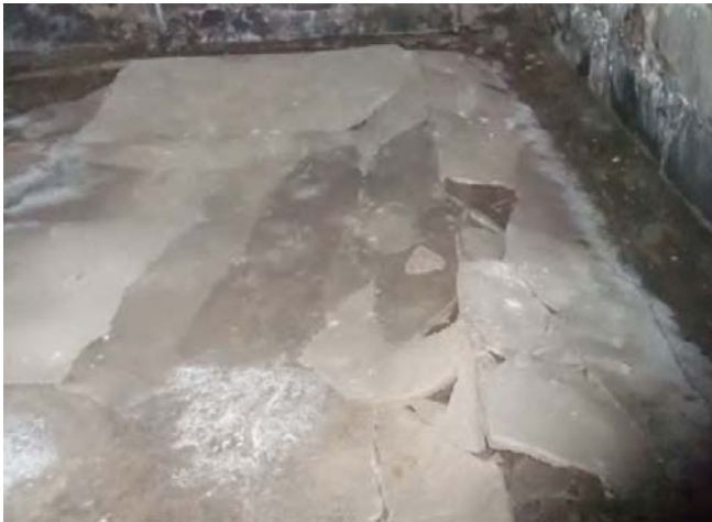
Photograph 1: Slab Heaving in Unheated Basement —So why didn't the walls collapse inwards and only the slab buckled upward? Easy, the ground beside the foundation wall was not wet, only the ground under the slab was wet. Another "ah ha" moment. You need wet soil for frost heave. Not only do you need wet soil, you actually need "frost-susceptible" wet soil. A miserable type of soil with an annoying distribution of fines. The size of voids in a soil determines its frost-susceptibility. More than 3% grains finer than 0.02 mm in diameter by weight usually are a problem.
